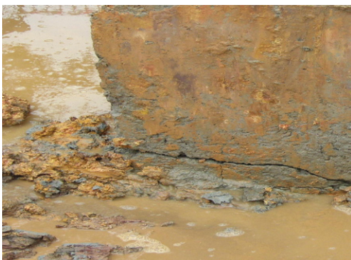
Visible cracks formed
